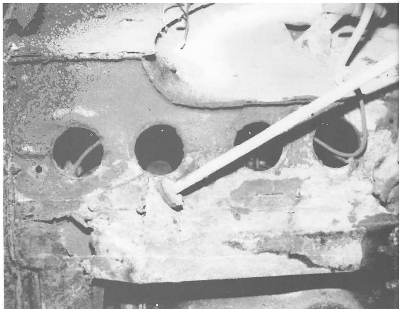
A badly rotted out and much repaired chassis leg. Even old MOT patches had been repatched.
